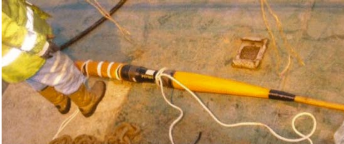
Figure 17-22: Damaged Cable Repair Joint on Cableship
