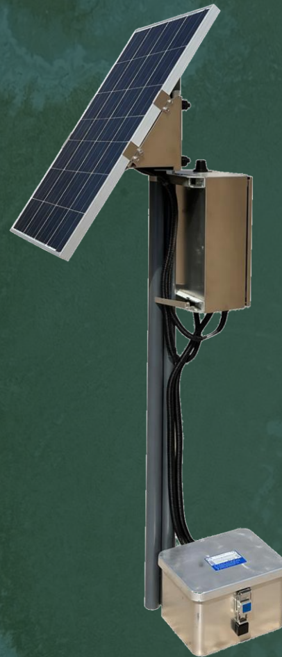
CO 2 Watch Onshore Station
