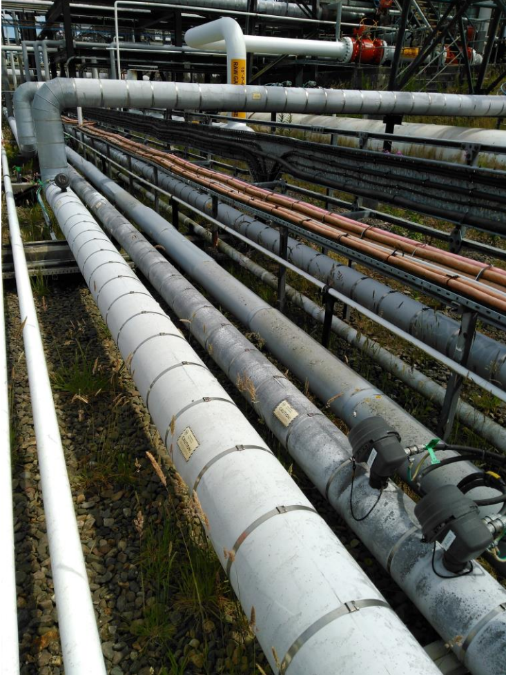
General View of Pipework in Track
